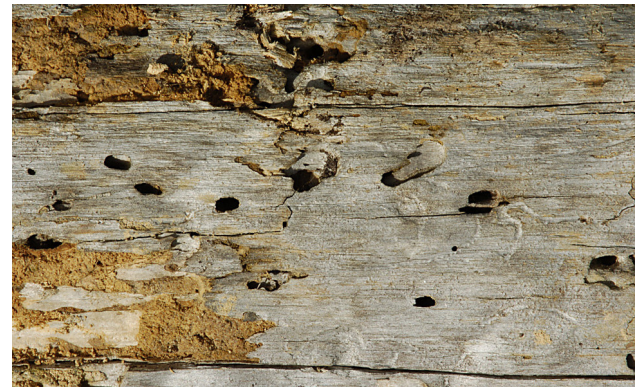
EHB emergence holes and blistering of wood
