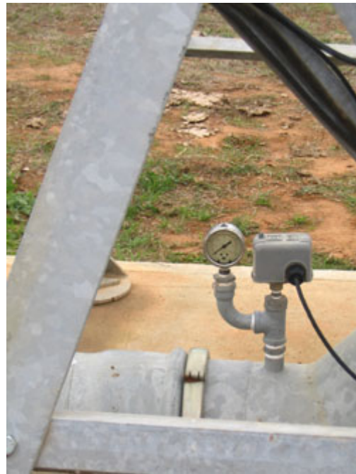
Figure 2 Check the pressure gauges
