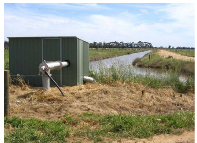
Figure 1 Centre pivot pump shed with suction from a drainage reuse sump
