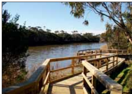
Project complete: replace the boardwalk and construct four fishing platforms on the south bank of the Tarwin River (two-year project funded for $115,000).
