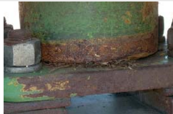
Organic matter lodged in joint
